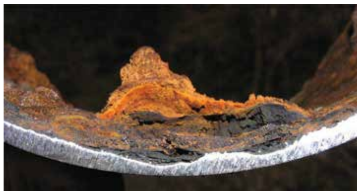
Figure 2. Classic example of pitting under deposits
